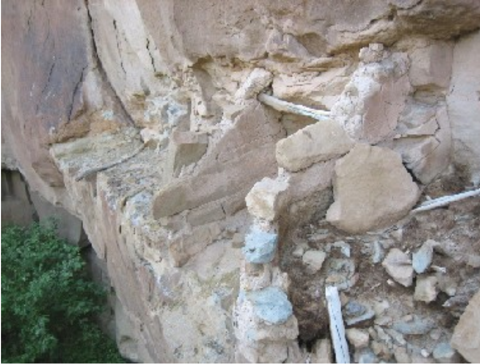
Figure 3.21: Lateral view of storage chambers at 42Em2441 (K.R. Barlow, courtesy of National Geographic Committee for Research and Exploration)
