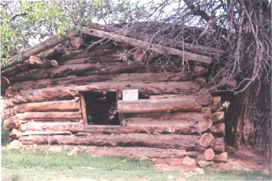
Figure 3.39: View of John Darioli/Joe Wing Cabin (42Em2875), as observed in 2002 (J.D. Spangler).
